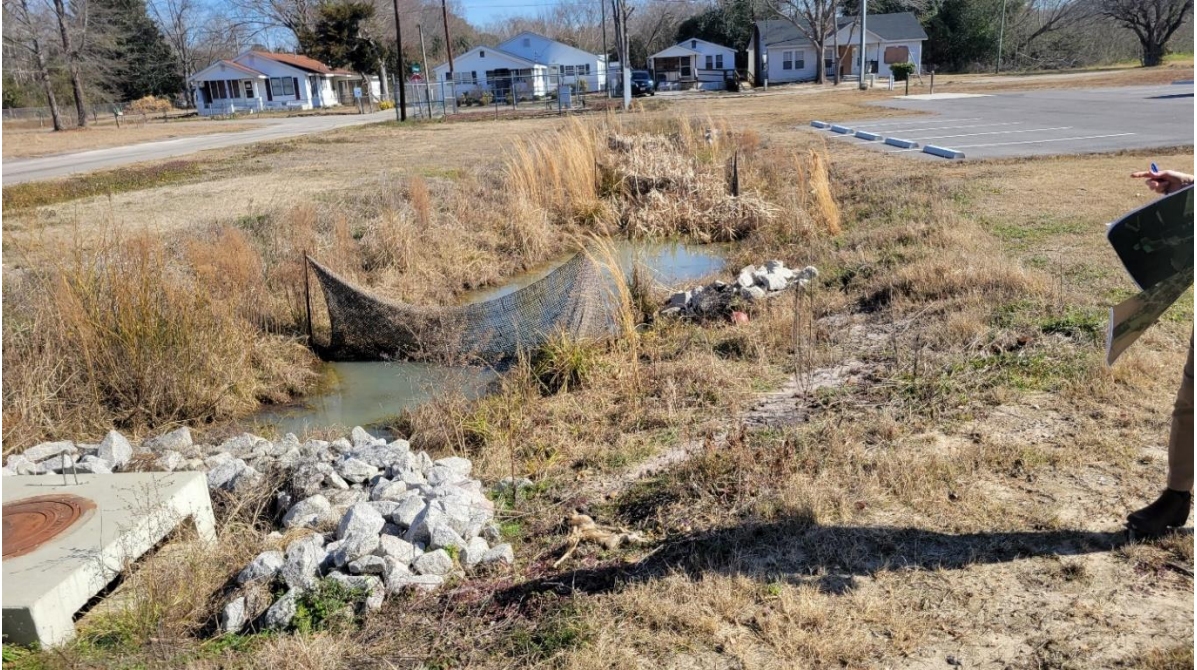
Figure 13. Stormwater Management Pond behind Museum
