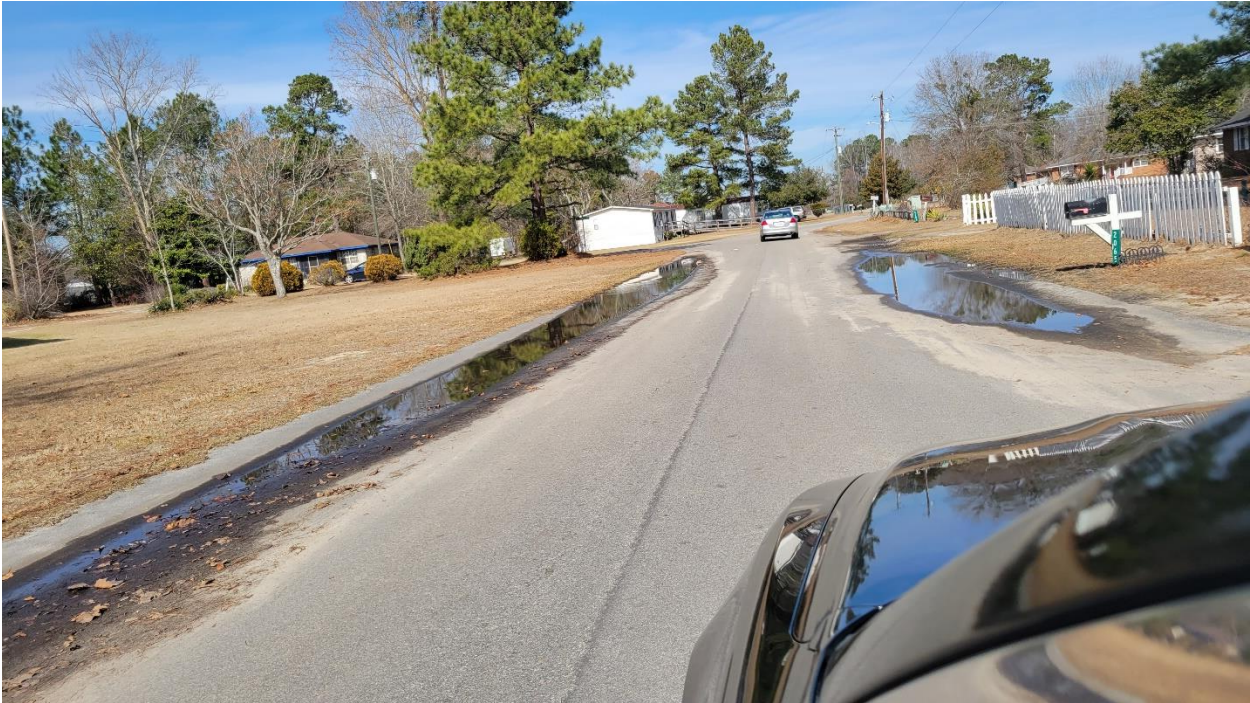
Figure 22. Typical Street Ponding along Avenue B
